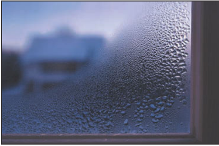
Condensation on the inside of a windowpane.
